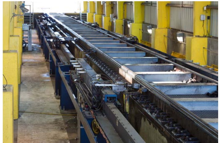
Ultrasonic wheel-defect detection identifies internal cracks or defects inside wheels on moving trains and reduces derailments caused by broken wheels.
