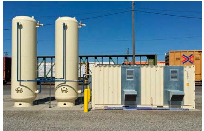
A new air compressor system reduces electricity and is 90 percent more energy efficient than air compressors used prior to installation.
