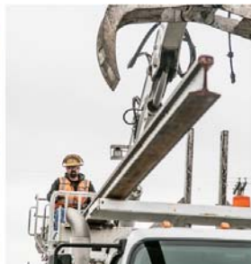
Automated Rail Unloading
